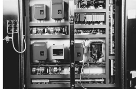
FIGURE 11.6 After—The panel now features a digital communications network (DeviceNet, in this case) that reduces wiring and increases flexibility.
