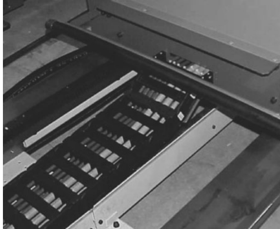
FIGURE 12.8 Cable between AGV track.
